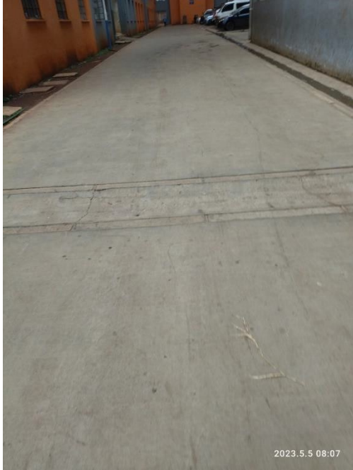
Figure 4.32 Trench in the middle of the road within the environment of the housing facility. (Source; Researcher, 2023)
