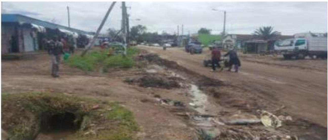
Plate 5.5: Eroded Road with a poor drainage system
