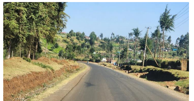
(f) Completed section of the upgrade showing erodible and unprotected embankment slopes (Author, 2023)
