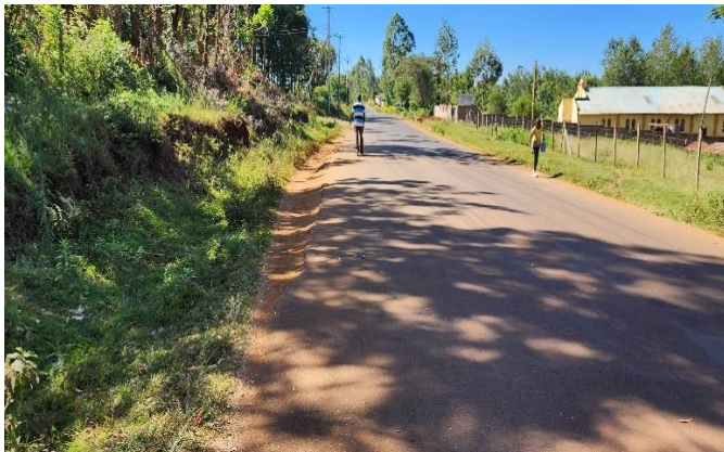
(a) Road start showing signs of edge subsidence, but the surfacing still intact (Author, 2023).
