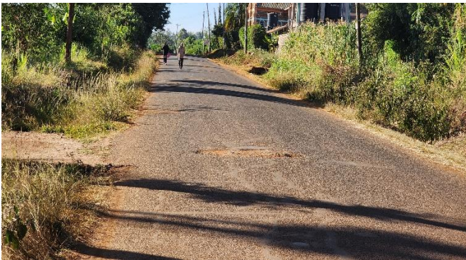
(a) Road start showing signs of failure by potholing. Overgrown vegetation also noted obstructing flow of water on the drainage system (Author, 2023).
