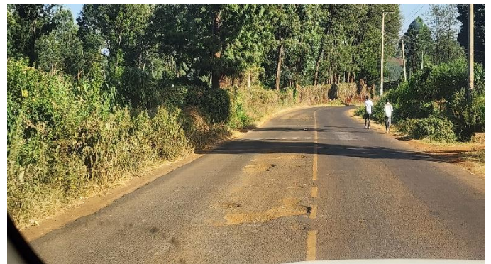
(b) Section showing continuous failure of the pavement by potholing. Inadequate drainage system noted (Author, 2023).
