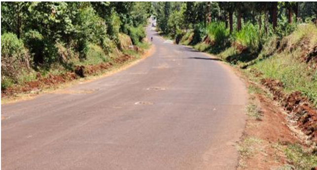
(c) Section showing the road geometry, drainage and surfacing. Asphalt surface intact on most sections, but poor drainage system noted even after routine maintenance. (Author, 2023).
