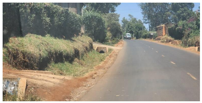
(d) Section offering good serviceability but poor maintenance showing on silted drains and culverts (Author, 2023).
