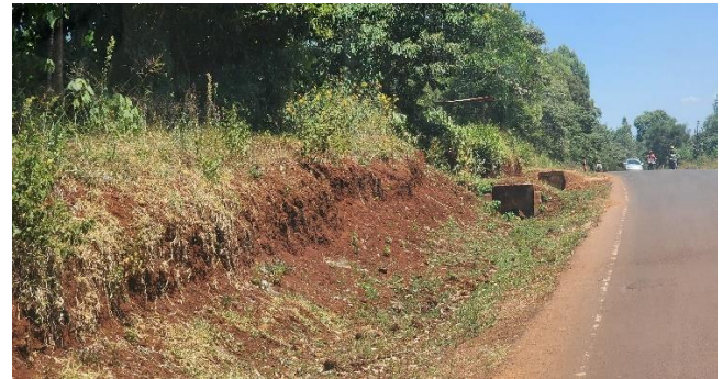
(d) Section showing unprotected slopes prone to erosion, leading to siltation of the drains and culverts (Author, 2023).
