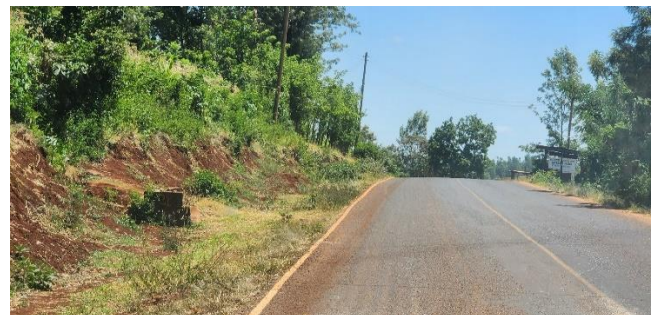
(d) Section showing unprotected slopes prone to erosion, leading to siltation of the drains and culverts (Author, 2023).
