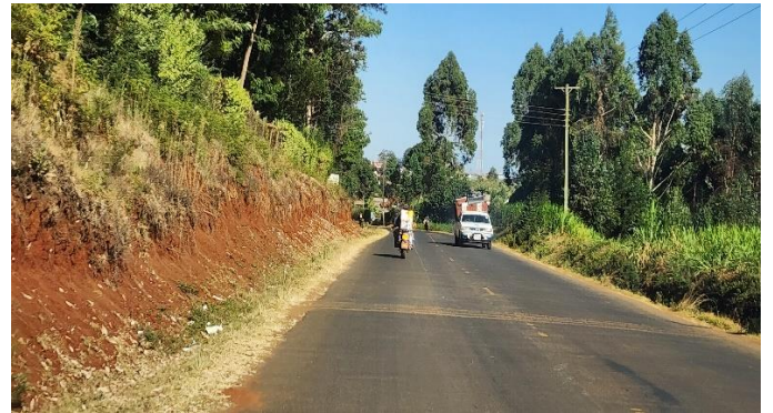
(b) Section showing the embankment slopes on the left with high erosion potential and already silted drainage system (Author, 2023).
