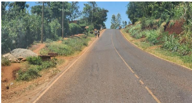
(a) Section showing the finished smooth surface. The drainage system was however not well defined (Author, 2023).
