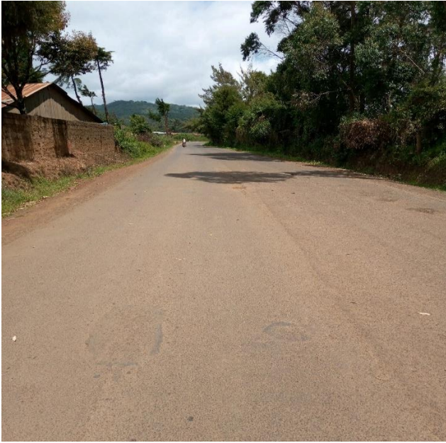
(a) Old pavement, at Km 0+010 where damaged surfacing had been repaired (Author, 2021)
