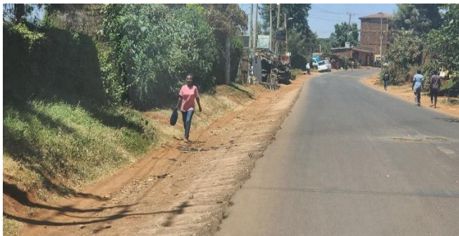
(a) Section of the road exhibiting failure by edge subsidence and potholing (Author, 2023).
