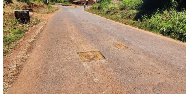
(b) Section showing pothole patching maintenance works in progress. The ride quality was rough on most sections (Author, 2023).
