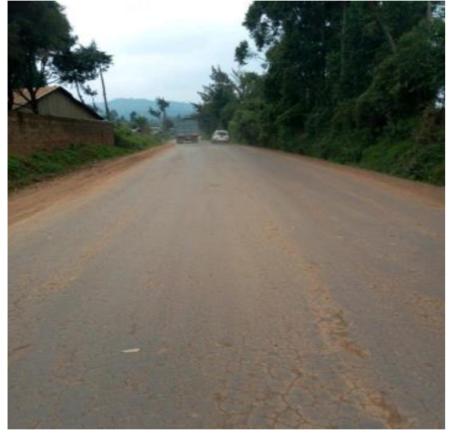
(b) Km 0+010 where asphalt layer has been damaged (Author, 2020).
