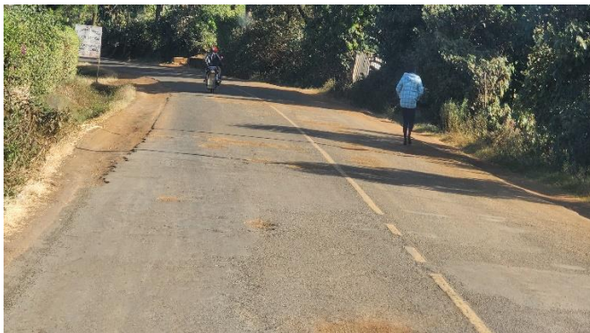
(a) Road start that was quite rough showing the continuing deterioration of the surfacing on that section (Author, 2023).
