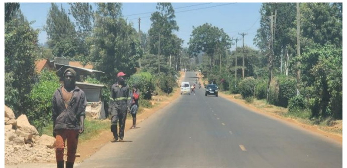
(b) Road section still in good condition and offering a smooth rideability (Author, 2023).
