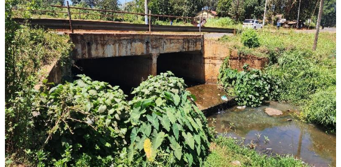
(b) Twin-box culvert in good operating condition, but water pooling was noted at the exit side of the structure. Poor routine maintenance noted. (Author, 2023).
