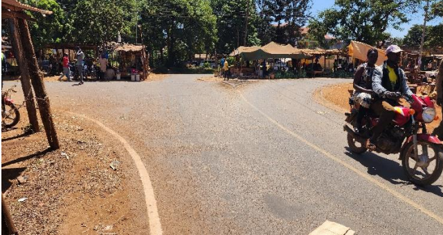
(a) Road start at Maragwa town. Asphalt surface intact, but poor drainage system noted (Author, 2023).
