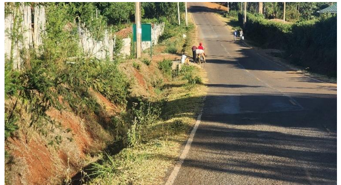
(b) Unlined drains with embankment slopes exhibiting high erodibility potential (Author, 2023).
