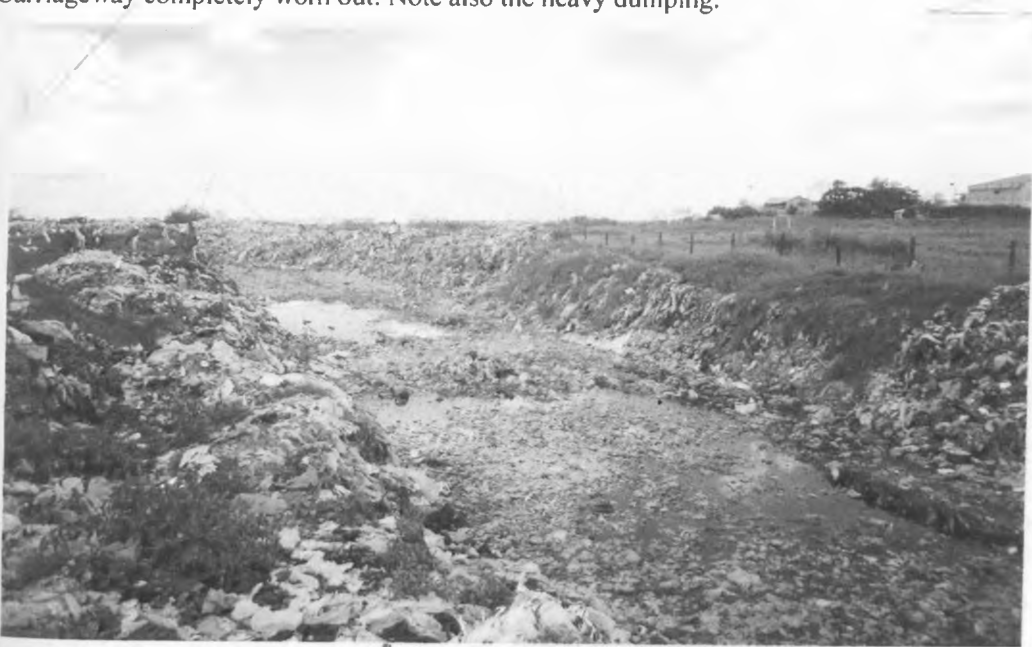
Plate 4.11: Remains of Northern Spine Road in Area 6 Carriageway completely worn out: Note also the heavy dumping.
