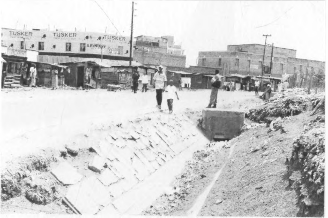
Plate 4.17 Silting in a Storm Water Drain Along the Northern Spine Road.
