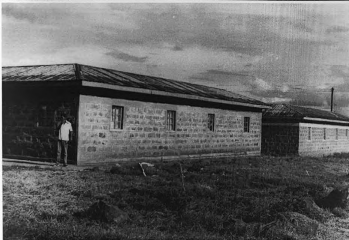
Residential houses opposite the factory with corroded iron sheets
