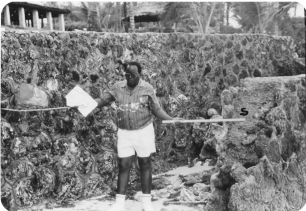
Plate 47 shows a thick vertical seawall (s) at Shanzu. A new seawall is inland of the failed seawall (s) (June, 1991; Photo by S. Langat).
