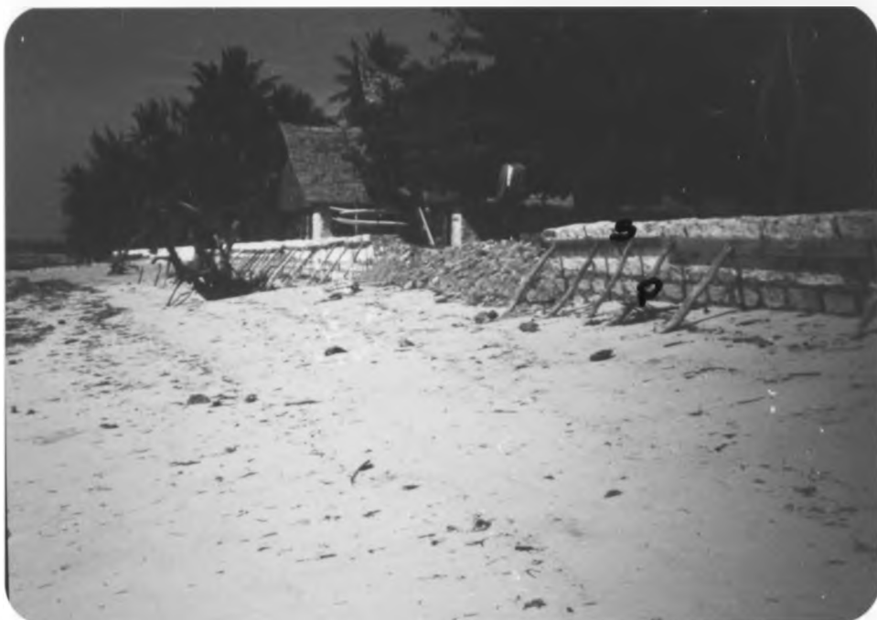
Plate 40 shows a seawall (s) at Kikambala. Wall is held in position by mangrove poles (p). This wall has however now fallen (September, 1990; Photo by P. Abuodha).
