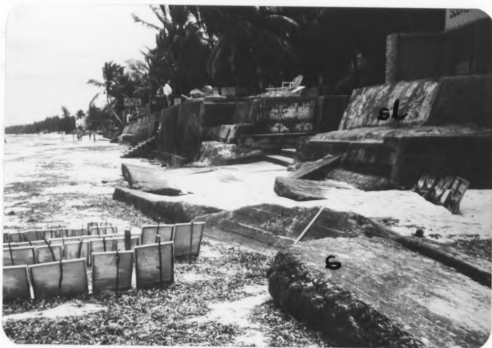
Plate 48 shows a thick seawall (s) at Bamburi. Note another seawall (sl) behind the failed wall (s) (September, 1990; Photo by P. Abuodha).
