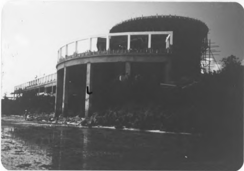
Plate 34 shows construction of property at the entrance to Tudor Creek. Note level (1) of high tide mark on the pillars (September, 1990; Photo by P. Abuodha.)
