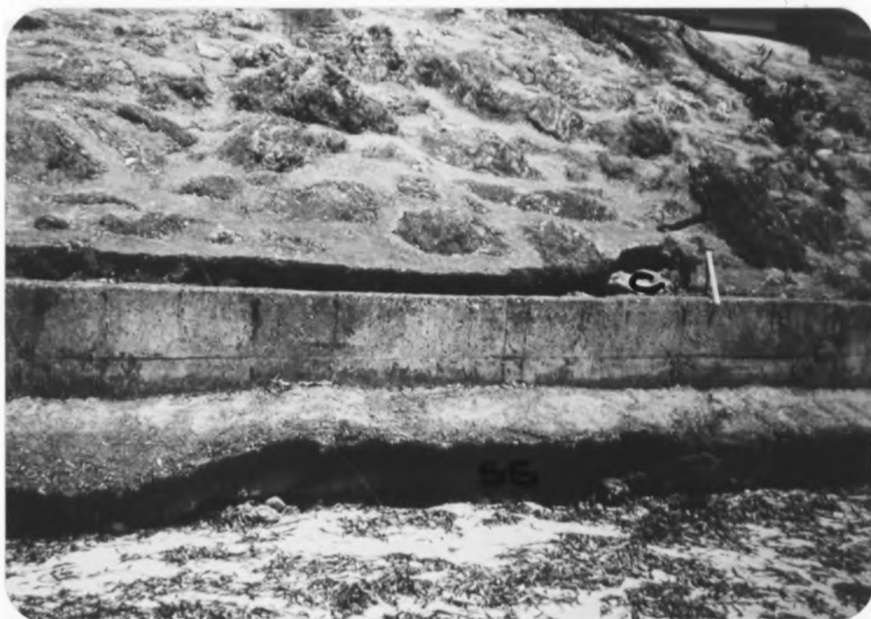
Plate 49 shows seawall along Nyali beach. Note crack (c) on the wall and the result of sediment scour (ss) beneath the wall (September, 1990; Photo by P. Abuodha).
