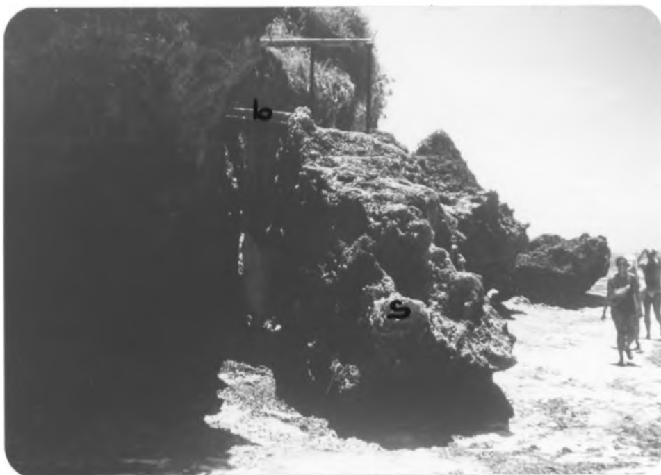
Plate 26 shows slab (s) failure has cut off the only bridge (b) access to the sea at Shanzu (September, 1990; Photo by P. Abuodha).
