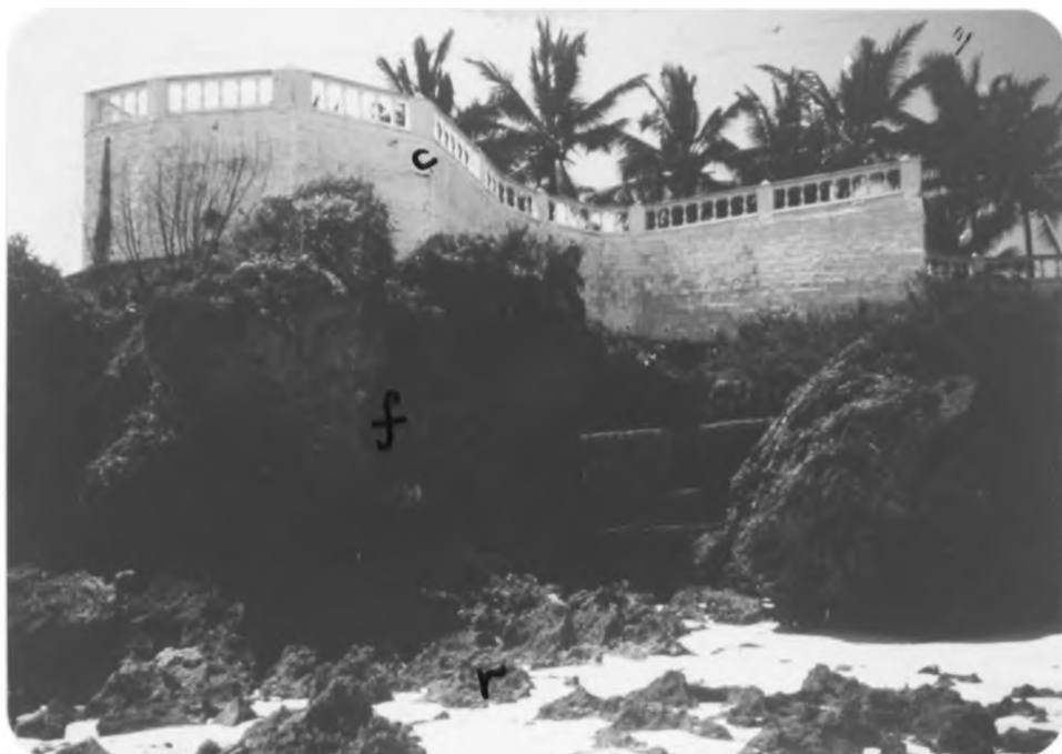
Plate 33 shows slab failure (f) leading to crack (c) on house wall at Leven. Note the exposed rocks (r) beneath (September, 1990; Photo by J. Abuodha).
