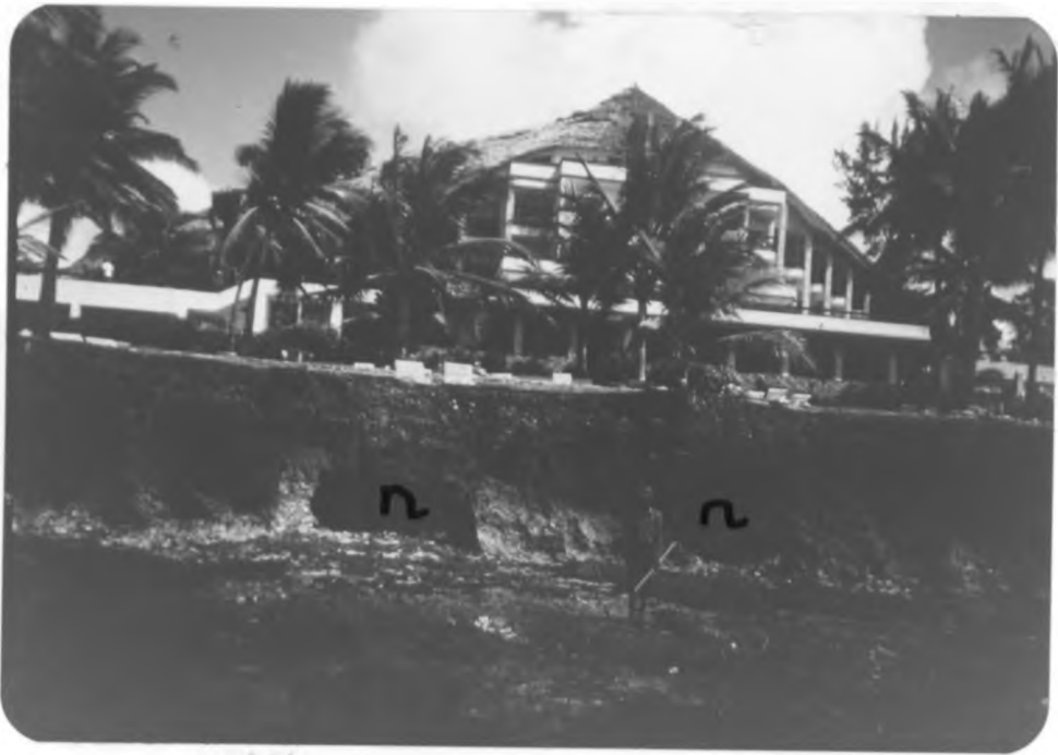
Plate 30 shows notches (n) developed beneath a beach hotel at Shanzu (September, 1990; Photo by P. Abuodha).
