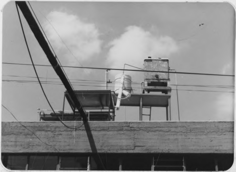
Plate 6. Thermosyphon Solar Water Heating System (front view).
