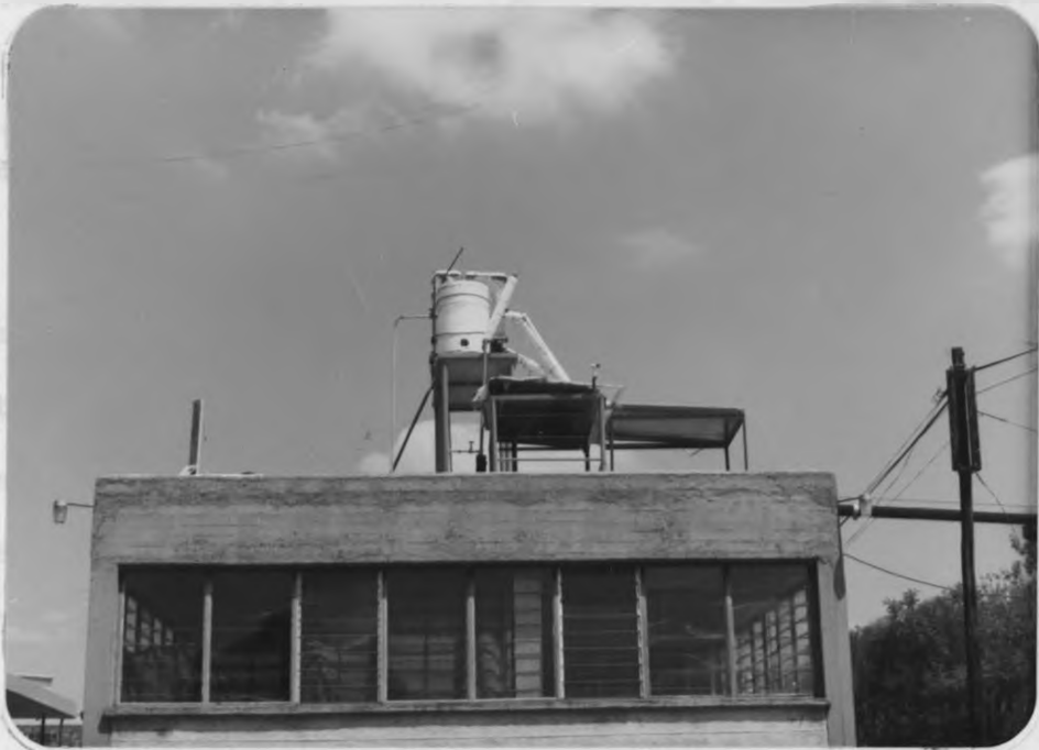
Plate 7. Thermosyphon Solar Water Heating System (side view).
