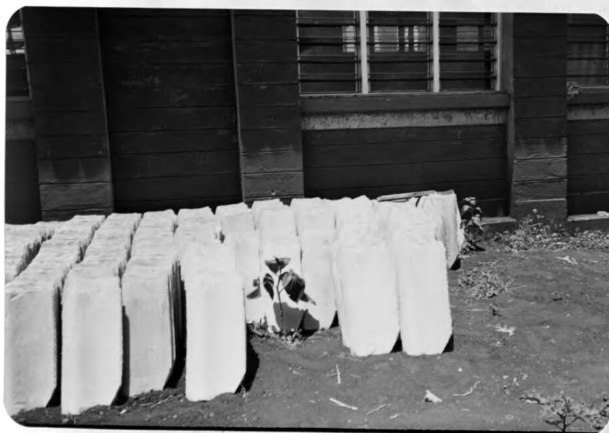
PLATE 4.12: KANGEMI, NAIROBI St. Joseph the Worker Parish, Kangemi, Nairobi. A classroom built of soil blocks with a cement rendering to which a brown pigment has been added.
