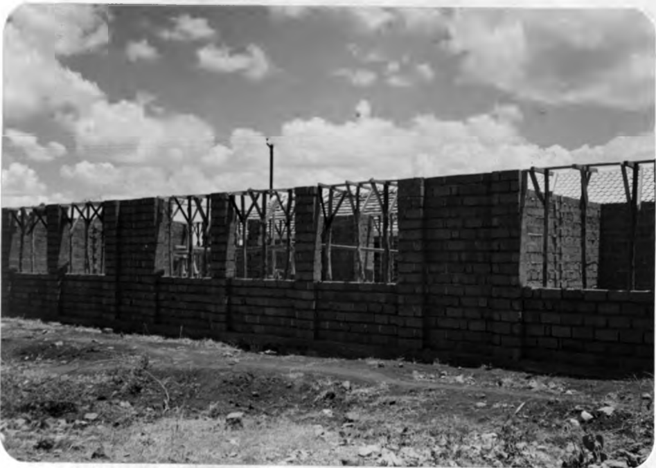
PLATE 3.8: KANGEMI, NAIROBI Classroom under construction at St. Joseph The Worker Primary School.
