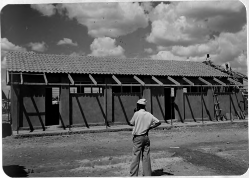
PLATE 3.9: KOROGOCHO, NAIROBI Classroom under construction at Korogocho Primary School. Note: The walls have been plastered.
