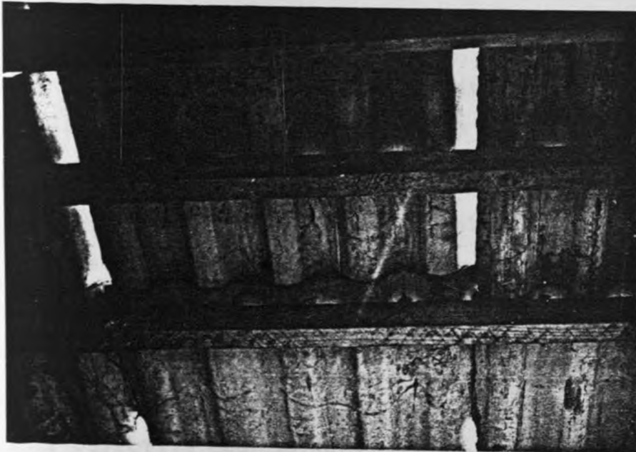
PLATE 4.3: JOINTS BETWEEN SISAL-CEMENT ROOFING SHEETS NOT YET FILLED WITH CEMENT MORTAR
