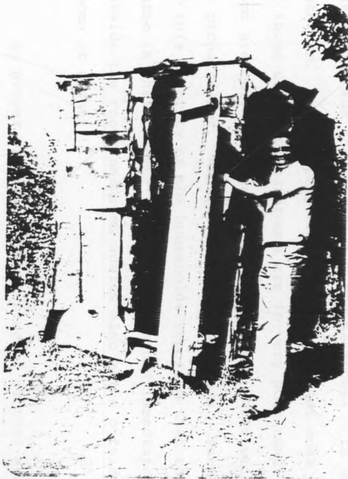
Plate 11: A - toilet without proper walls, roof and floor.
