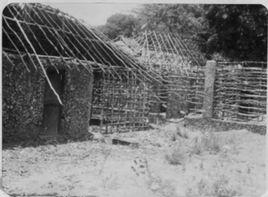
Plate 1: A swahili house under construction in Maweni. The finished wall is of "mtomo" mud.
