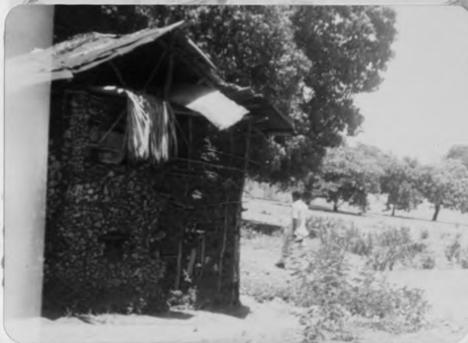
Plate 8: Some units are completely beyond repair, like this utility store near Barani.
