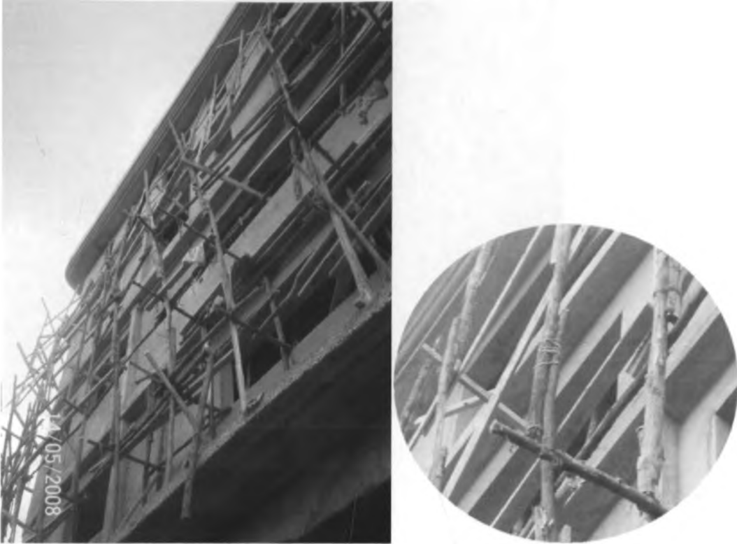
Plate 4. 3 The unsafe scaffolding used at some of the sites
