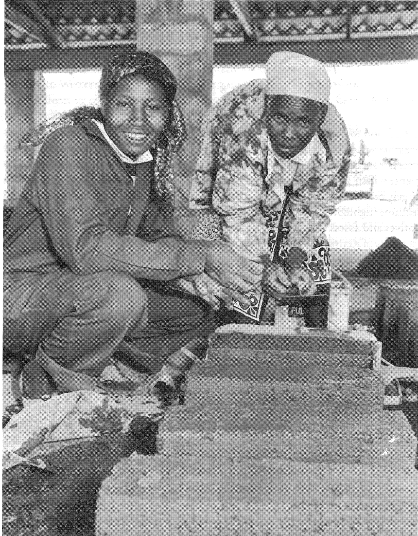
Women's self-help groups increasingly work to provide members with skills and income, sometimes in nontraditional areas. Under contract with the African Housing Fund, members of the Kayole Women's Self-Help group in Nairobi produce building materials, such as cinder block, and work in construction.
