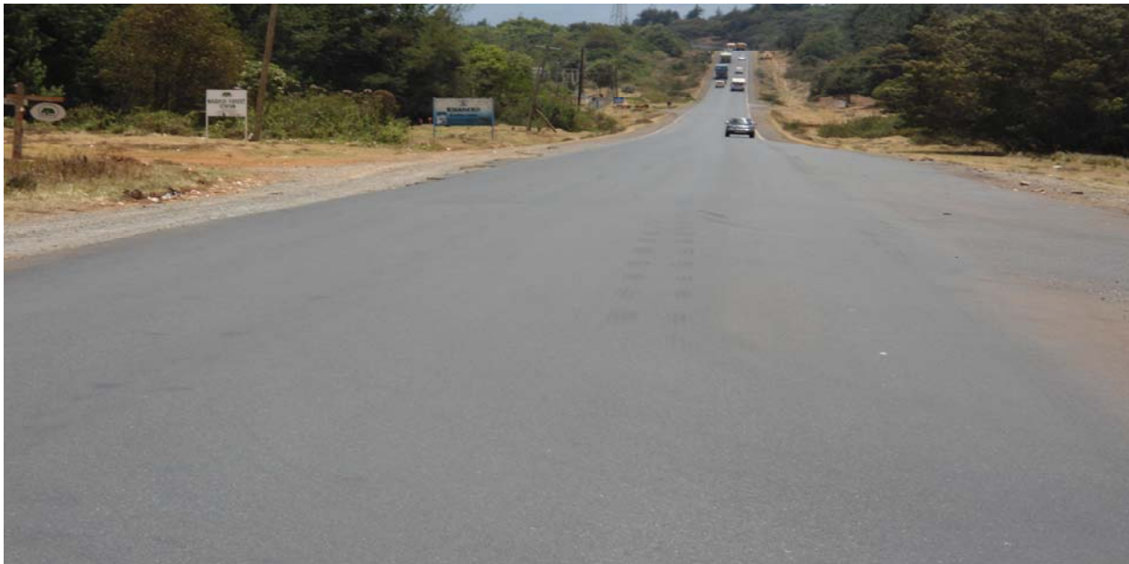
Figure 1.4: A flat section of the road just before the start of the worn out climbing section above
