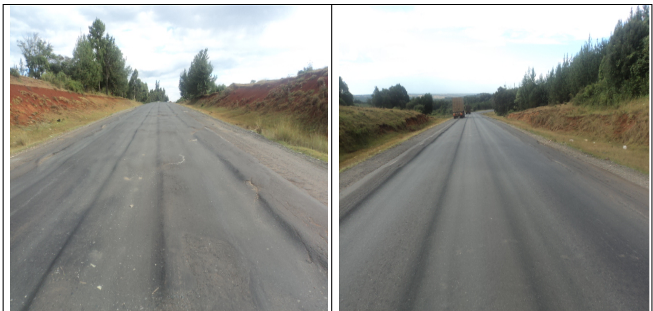
Figure 1.3: A section of the worn-out road shoulder of Northern Corridor (A104, Timbora)
