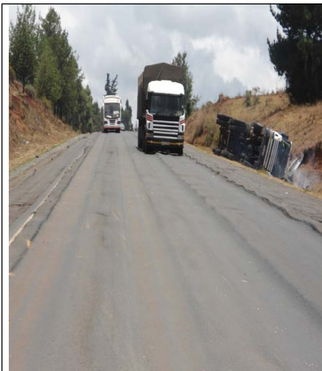
Poor pavement conditions on the section has been a key cause of accidents.
