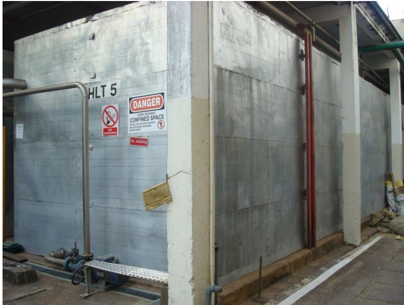
Photograph 4.1: Hot water storage tank (HLT 5)
