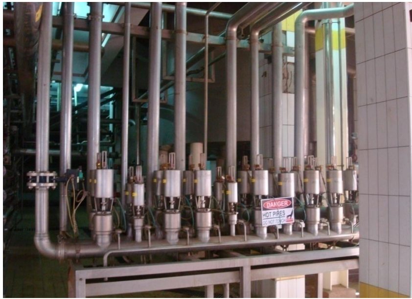
Photograph 4.2: Hot water distribution pipes and valves
