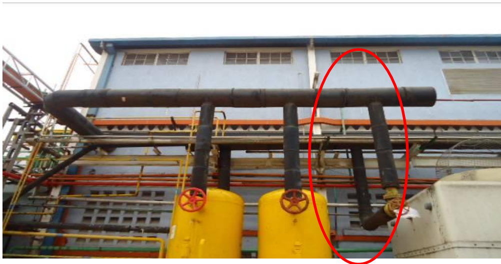
Figure 4-30: unused redundant pipes and oversized pipes
