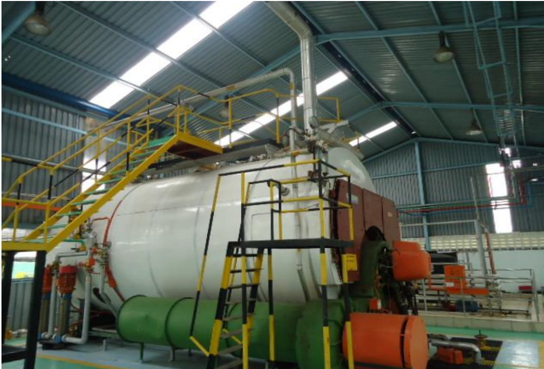
Figure 2-3: Unilever packaged boiler (2010)
