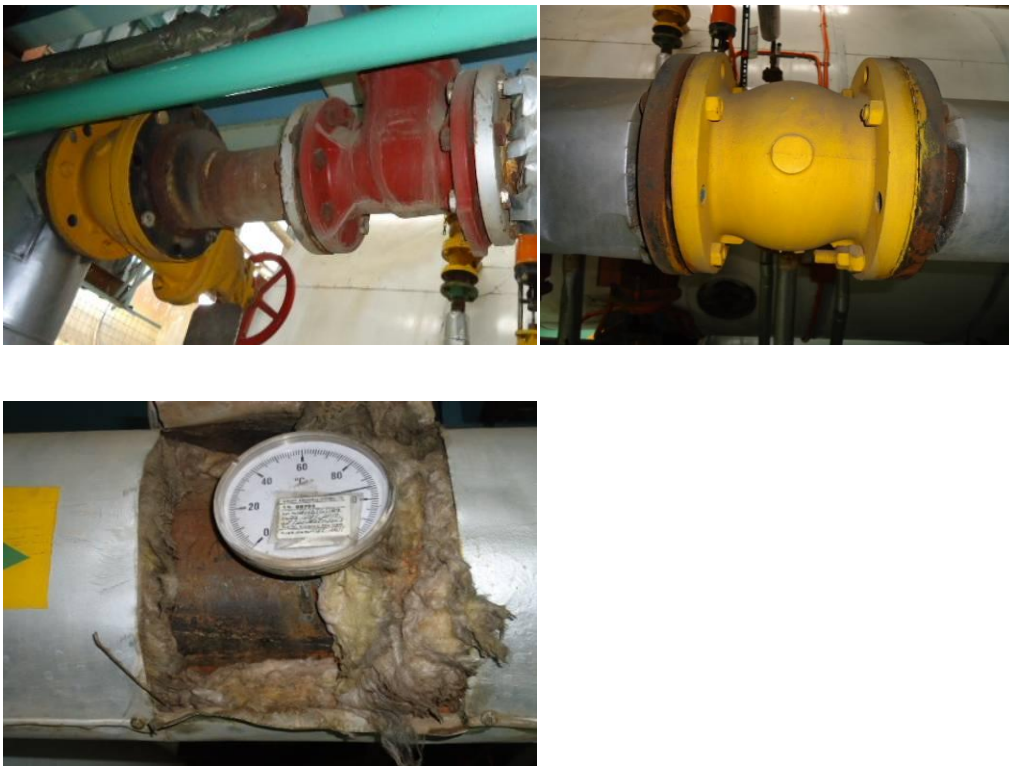
Figure 4-14: Unlagged Pipes, Valves and gauges
