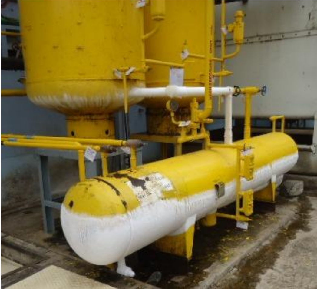
Figure 4-29: Unlagged Sections of the Ammonia Receiver Leading to Icing
