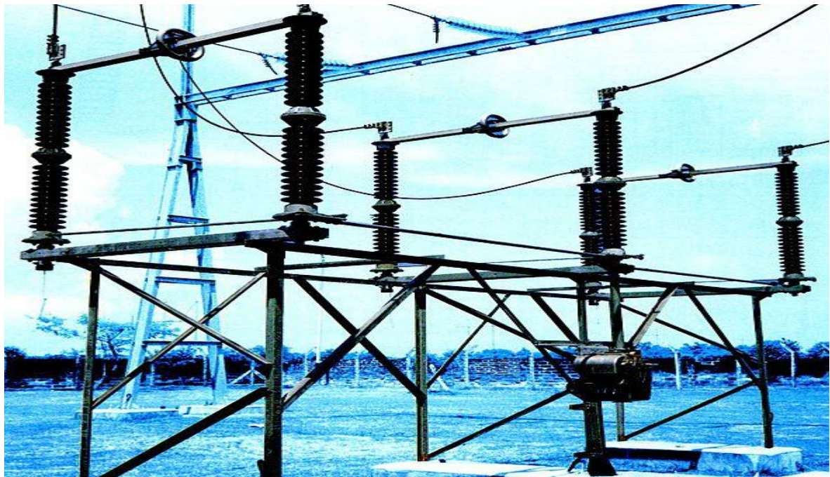
A high-voltage disconnect switch used in an electrical substation. Such switches are used mostly to isolate circuits, and usually cannot break load current. High-voltage switches are available for the highest transmission voltages, up to 1 million volts. This switch is gang-operated so that all three phases are interrupted at the same time
