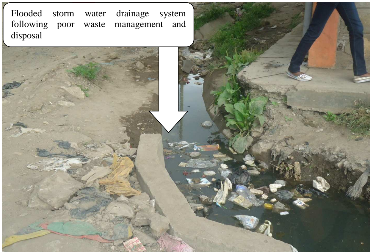
Plate 5.5: Flooded Storm water drainage.
