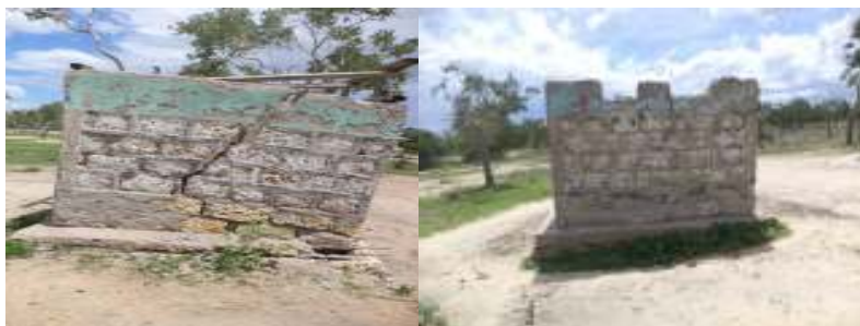
Fig 4.2 School toilets damaged by floods
