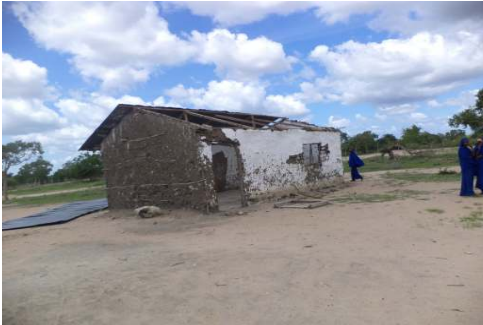
Fig 4.7 A classroom damaged by floods
