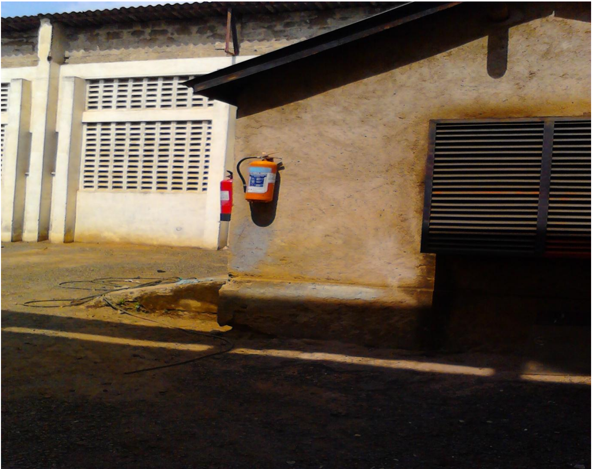
Fire extinguishers fitted on the wall of a commercial building in Kisumu's CBD
