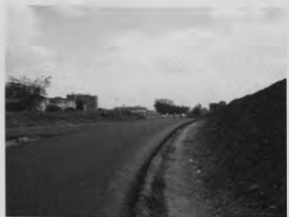
Figure 4.42 – Site III west side facade and the slip road on its last stage of construction. Source: Author, 2013.
