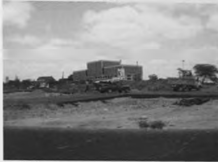
Figure 4.43 – Slip road already on use and still under construction. Area taken from site III. Source: Author, 2013.
