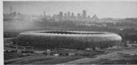
Figure 2. 16 – The Stadium under construction. Source: Official Website of the city of Johannesburg, 2010.
