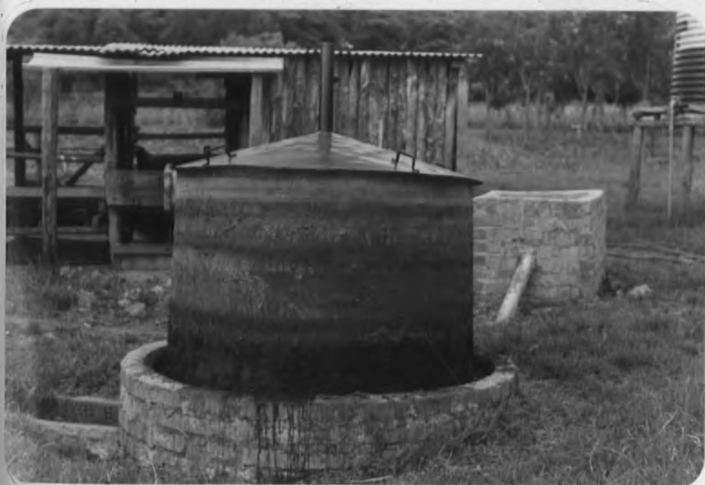
Plate 29: Digester and gas holder
