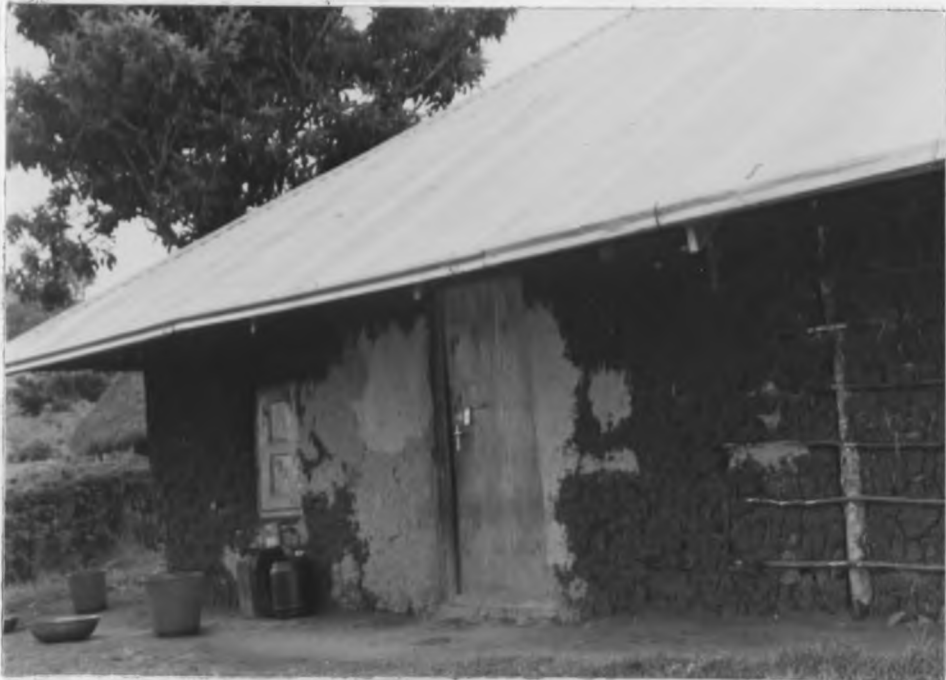
Plate 4-9: A Poorly maintained GCI Kisii house.
