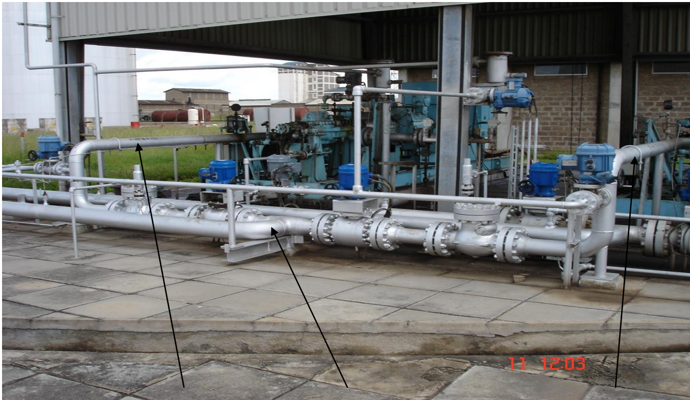
Discharge pipe 1 joint discharge pipe for two pumps Discharge pipe 2
