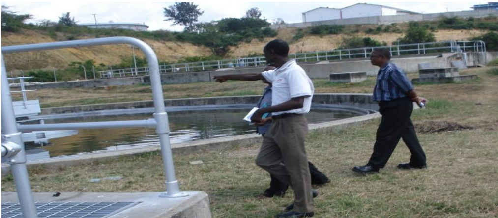
Figure 2. 4: Final settlement tanks
