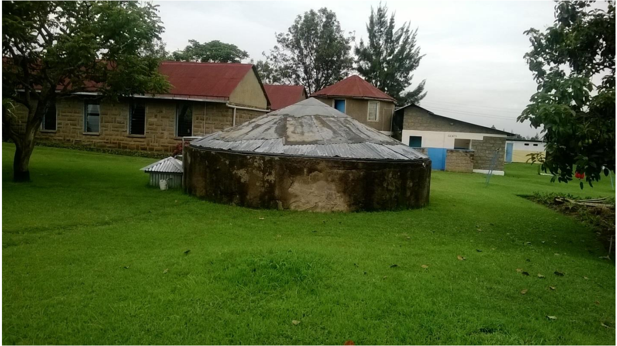
Plate 9: Rain Water Tank OR/010/14
