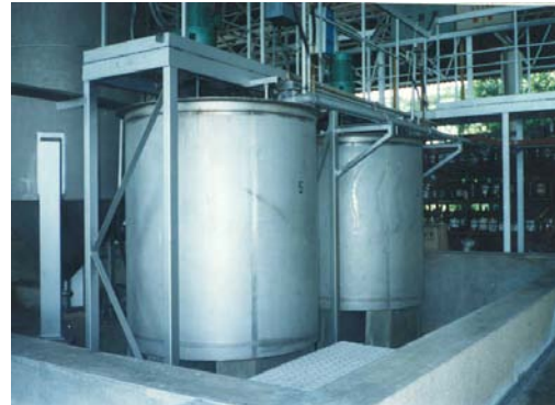
Low-Level Aqueous Effluent Treatment Plant
