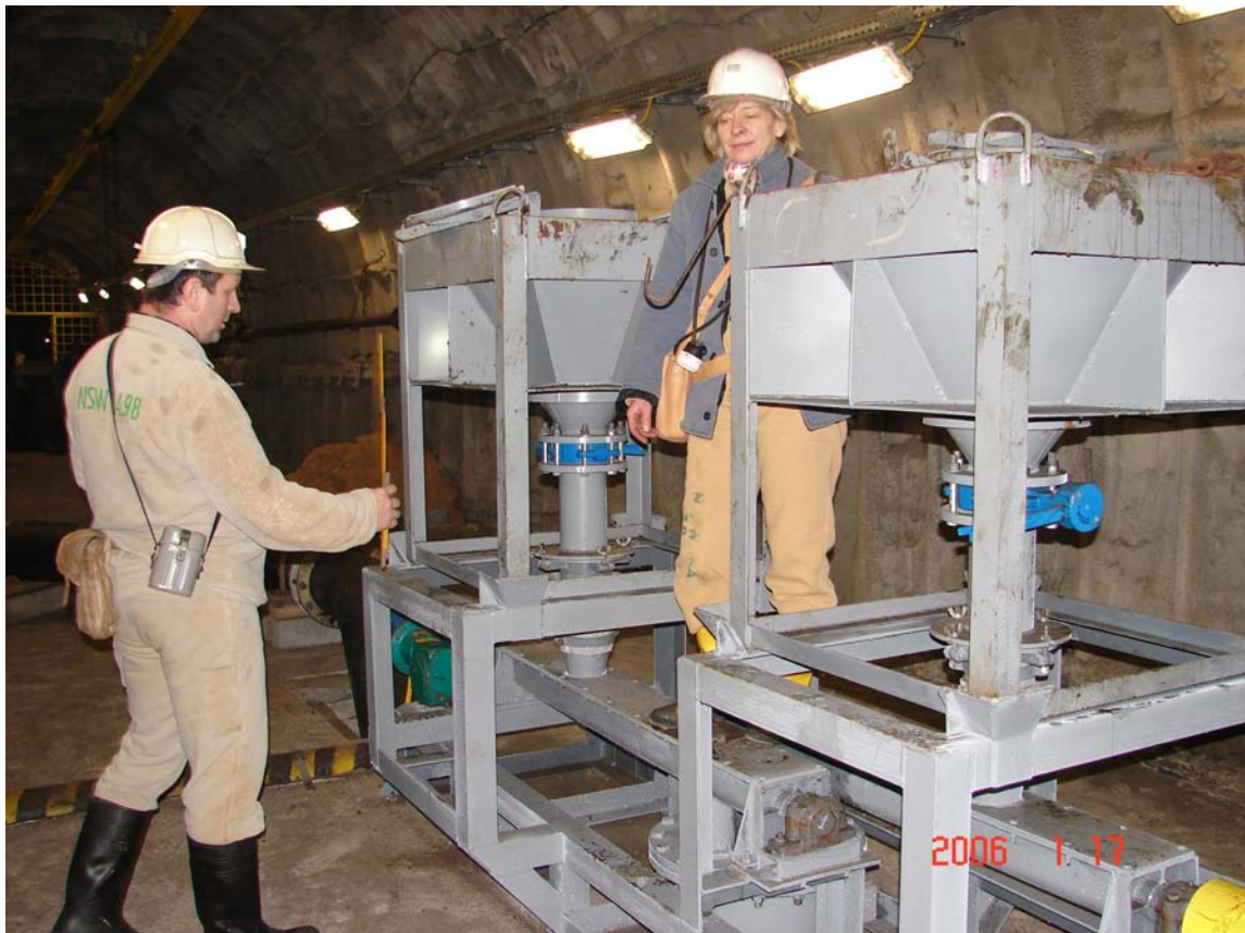
FIG.2. View of the purification station (2) in Ziemowit Colliery – feeders of BaCl_2
