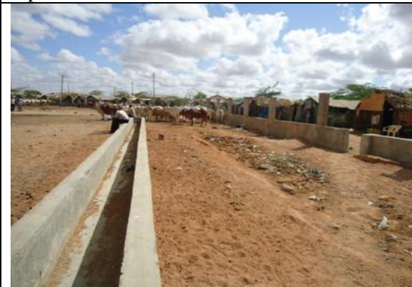
Picture from a follow-up visit showing new water trough and wall under construction separating food “kiosks” from market.
