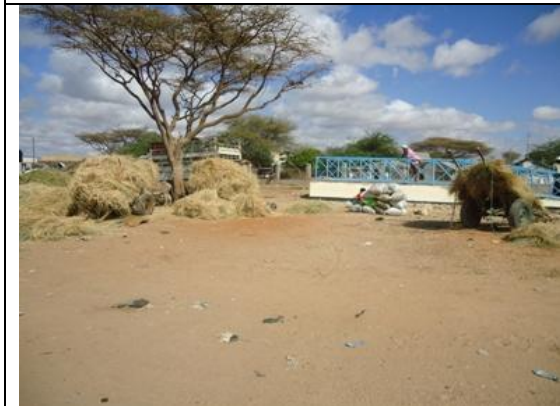
Picture from a follow-up visit showing new metal-sided loading ramp under construction and feeds on sale.
