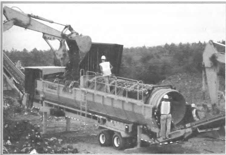
Plate 2.7: Trommel screen used for effective waste screening Source: Perdido LFM report 2008
