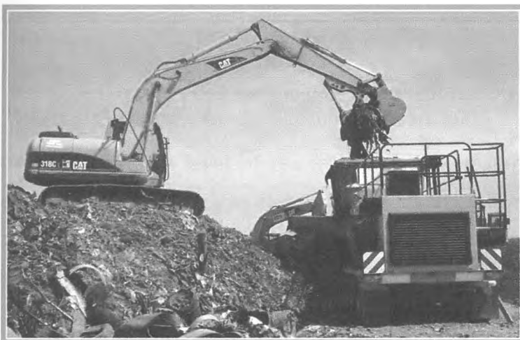
Plate 2.8 : Excavator feeding the excavated waste to the shredder Source:- Perdido LFM Report, 2008
