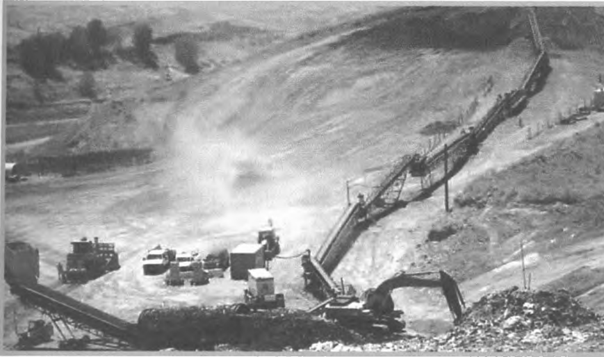
Plate 2.9: Conveyor belt system for soil transportation Source:- Clovis city, for Clovis Mining Report, 2005
