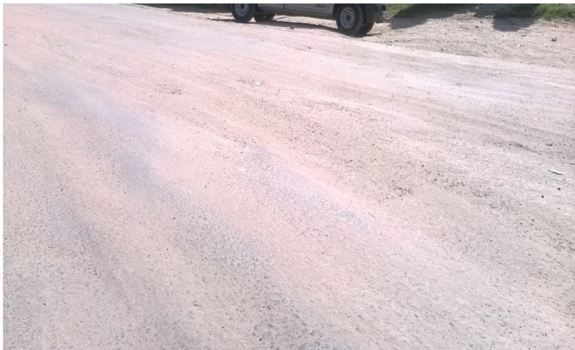
Plate 21: Loose Gravel on the Surface of the Road along Kasarani, Warren Road
