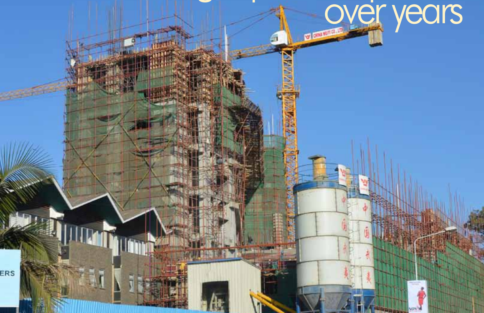
View of the ongoing construction of the University towers from Harry Thuku Road.
