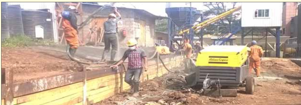
Laying the foundation of the ongoing construction of the University of Nairobi Towers.
