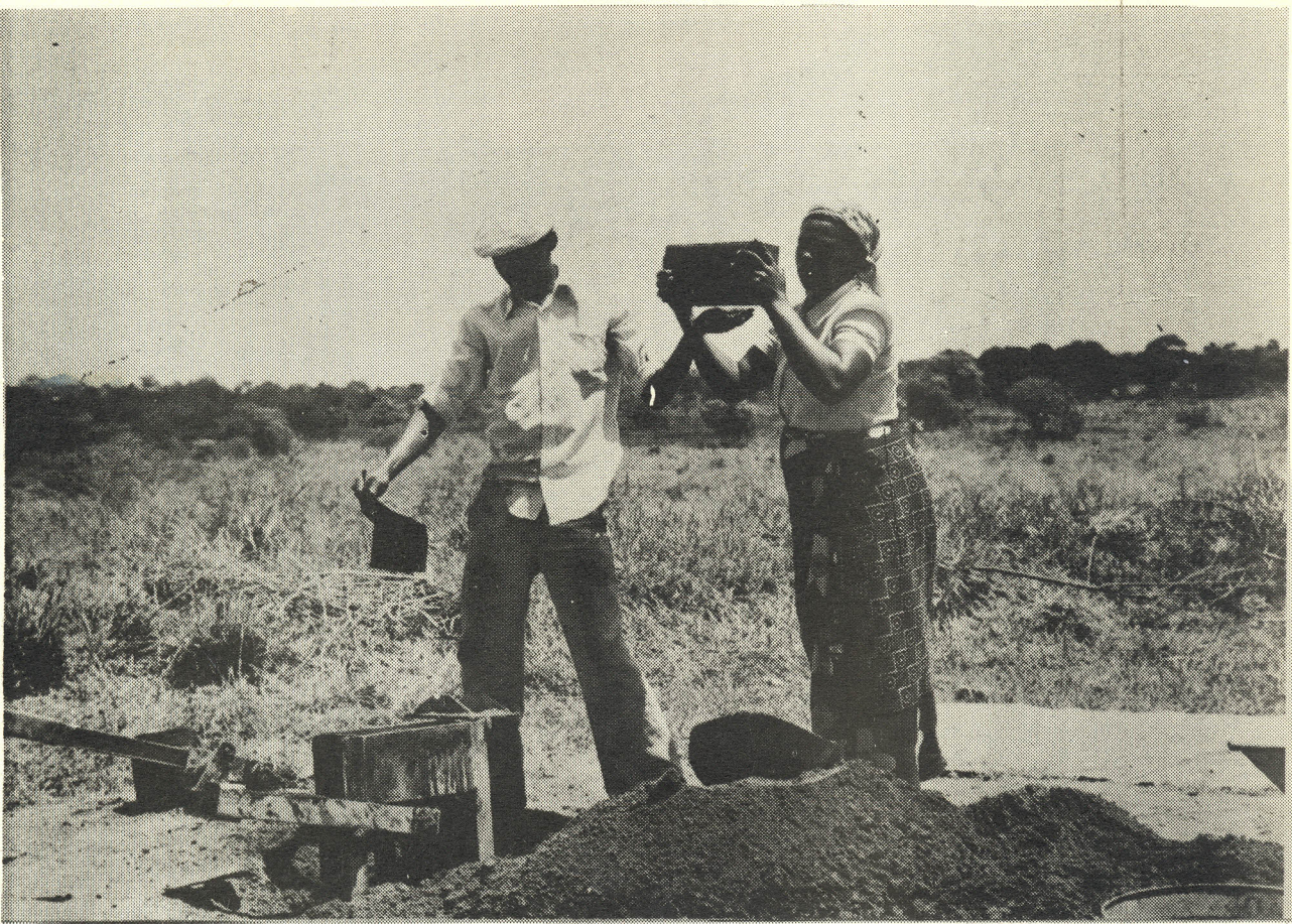
35. Immediately after compression the mud-block has its own shape and can be handled carefully as a solid.
