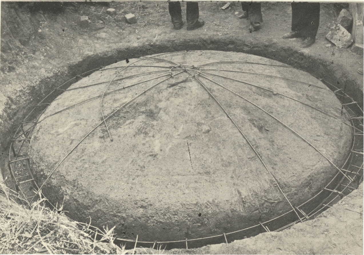
42. The underground ferrocement watertank: digging a trench, shaping the dome and placing the reinforcement.
