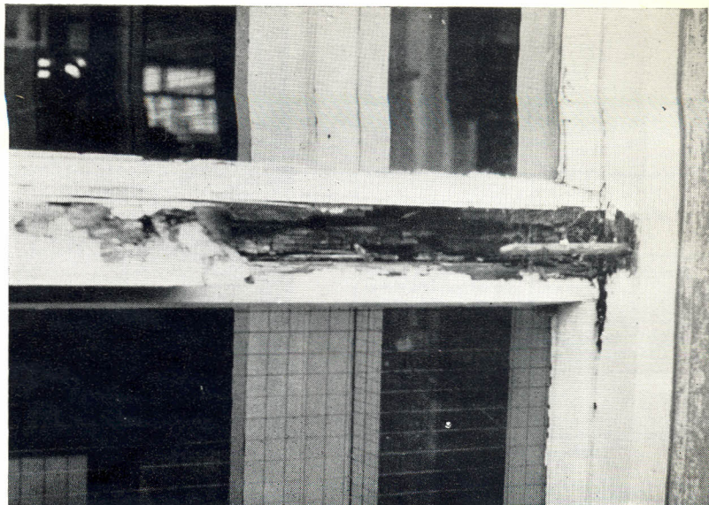
Fig 3 External part of mullion/transom joint held by nail. Result—water penetrates freely once the paint film is broken. Failure through decay began after three years' service
