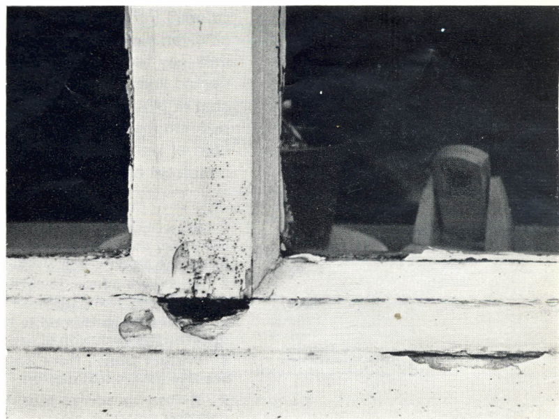
Fig 4 Gap left beneath tenon in joint between stile and cill or, in this case, between lower rail of main frame and base of mullion. Result—void for collection of moisture and eventual decay
