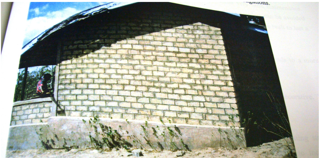
Fig. 3.2: Effect of high humidity on timber (fascia board) - no effect to SSBs
