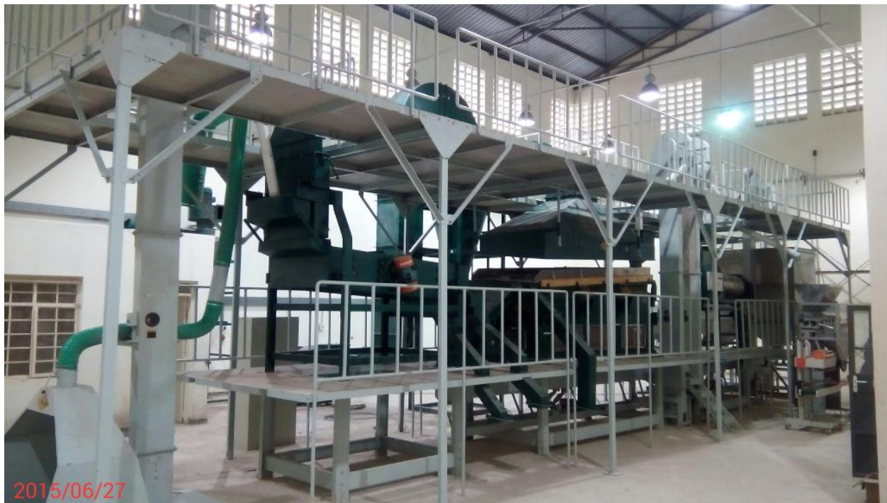
Installation of seed processing machines is complete
