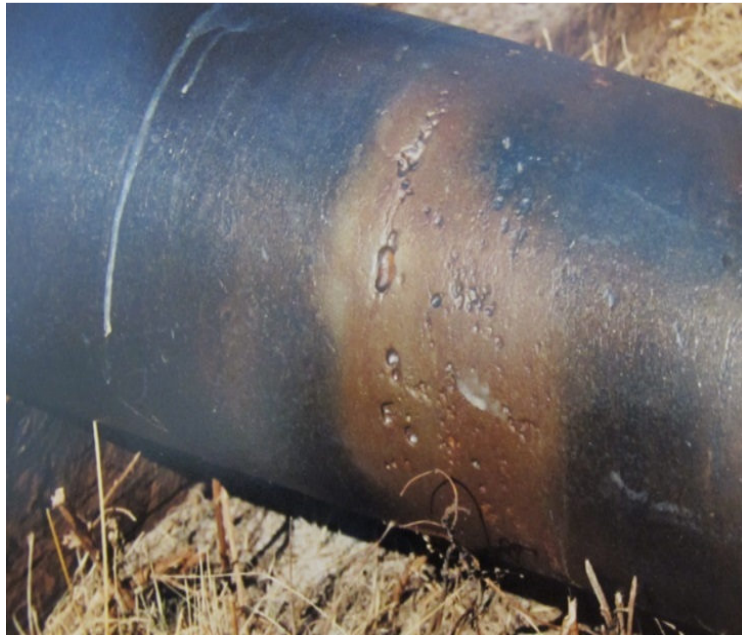
Plate 4-2: Corrosion band located from 3'5" from end 9A
