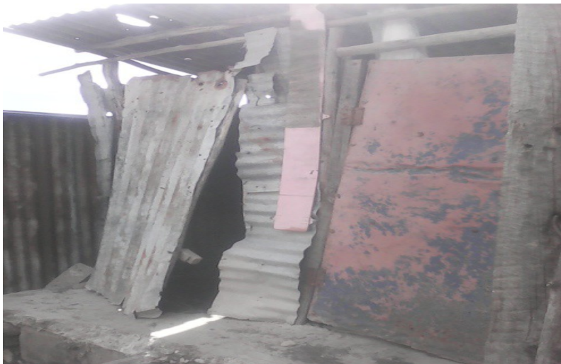
Plate 4.1 toilets that needs repair but still in use
