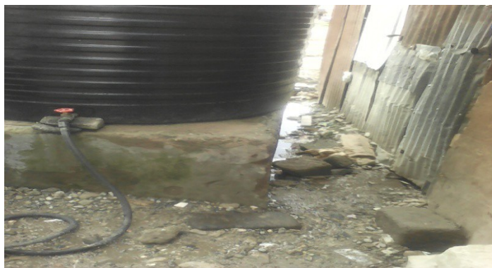
Plate 4.8 water point risk of contamination
