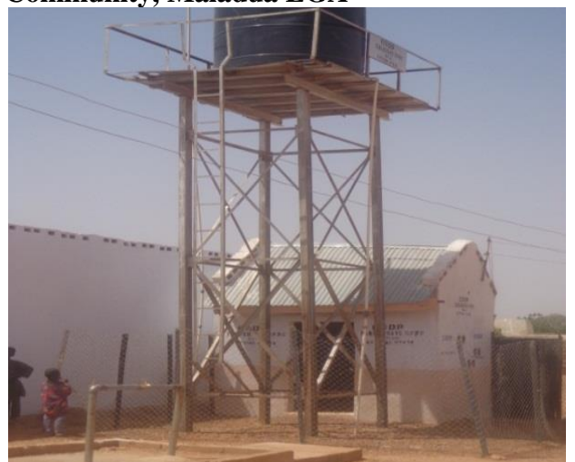
Plate 5.13: A Non-Functioning Motorised Borehole Constructed Under World-Bank Funded Project at Gwajo Gwajo Community, Maiadua LGA
