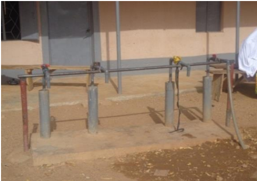
Plate 5.6: Pay-Per-Fetch Water Selling Point constructed by a Private Investor at Kofa Community, Kusada LGA
