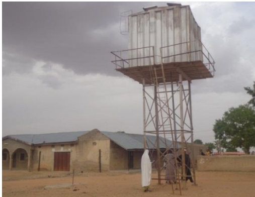
Plate 5.34: An Example of an Abandoned solar powered Borehole at Maigora Community, Faskari LGA
