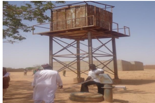
Plate 5.37: A Handpump Abandoned due to inability of the Community to be Funding the Cost at Kuraye Community, Charanchi LGA
