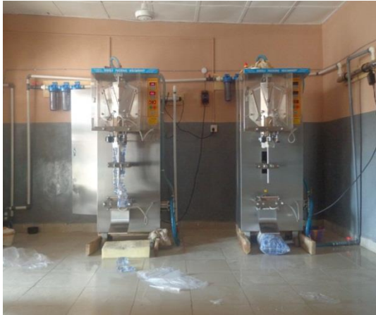
Plate 5.40: Sachet Water Making Facilities of a Private Firm at Kofa, Kusada LGA
