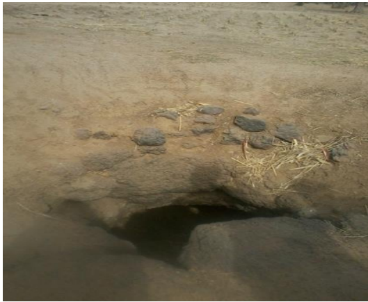
Plate 5.28: An Example of an Open Well at Mallamawa, Matazu LGA, Damaged through Collapsing of its Sides
