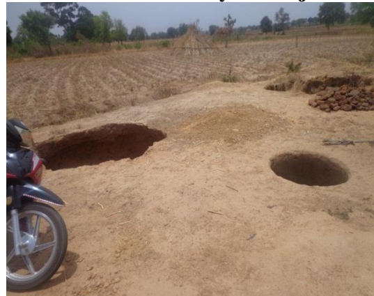
Plate 5.43: Changing location of a collapsed well within the same area at Tudun Jae Commonuty in Danja LGA
