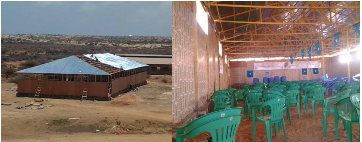
The Kismayu University delegates conference hall under construction funded by Jubbaland businessmen. Photo source: Radio Kismayu dated 24 February,2013
