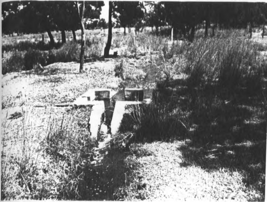
Plate 10: Aguthi Water Canal Division box
