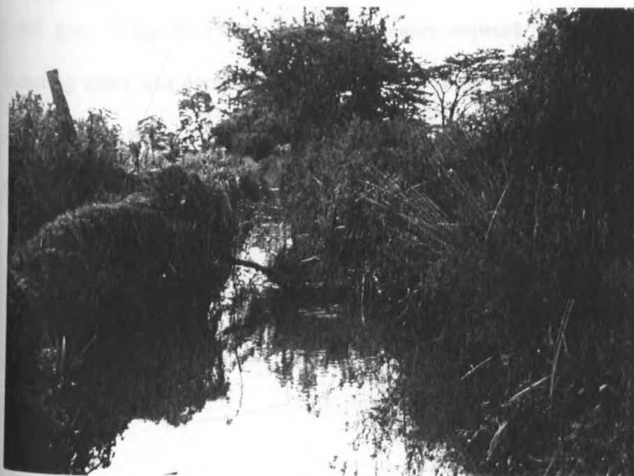
Plate 9: A canal section with distorted shape in Thome
