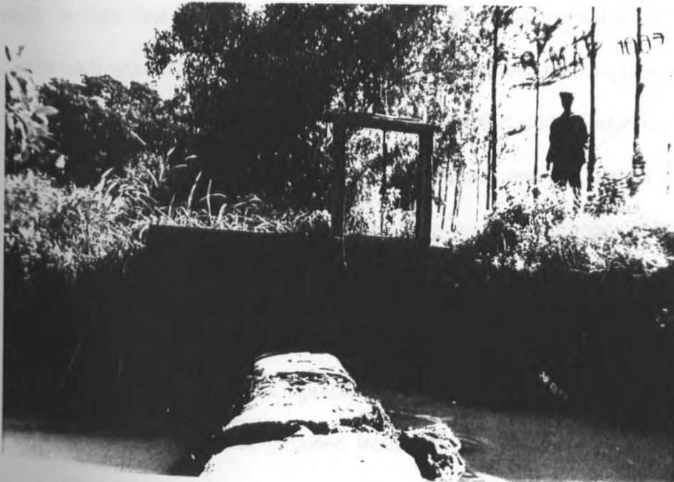
Plate 1: Cracked weir of Matanya canal intake point
