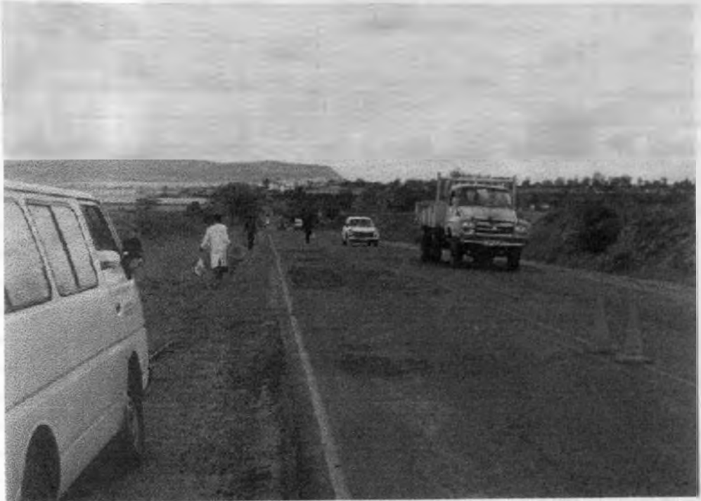
Plate A3.9 Test site ES6 showing ruts and cracks
