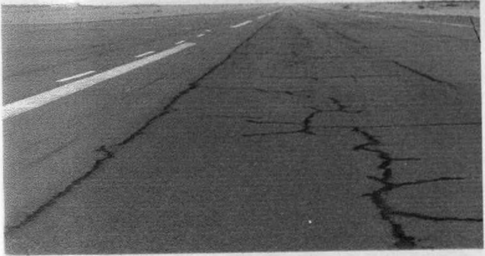
Plate A4.1 Pavement cracking on the runway
