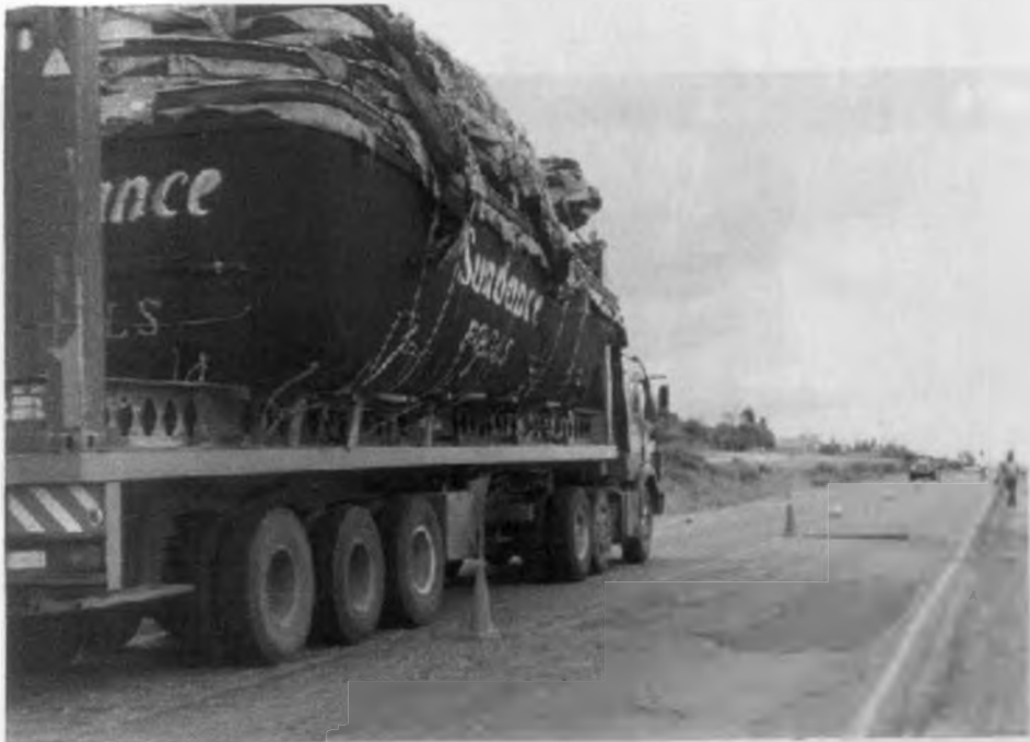
Plate A3.8 Test site ES5 with heavy axle loads, cracks and ruts
