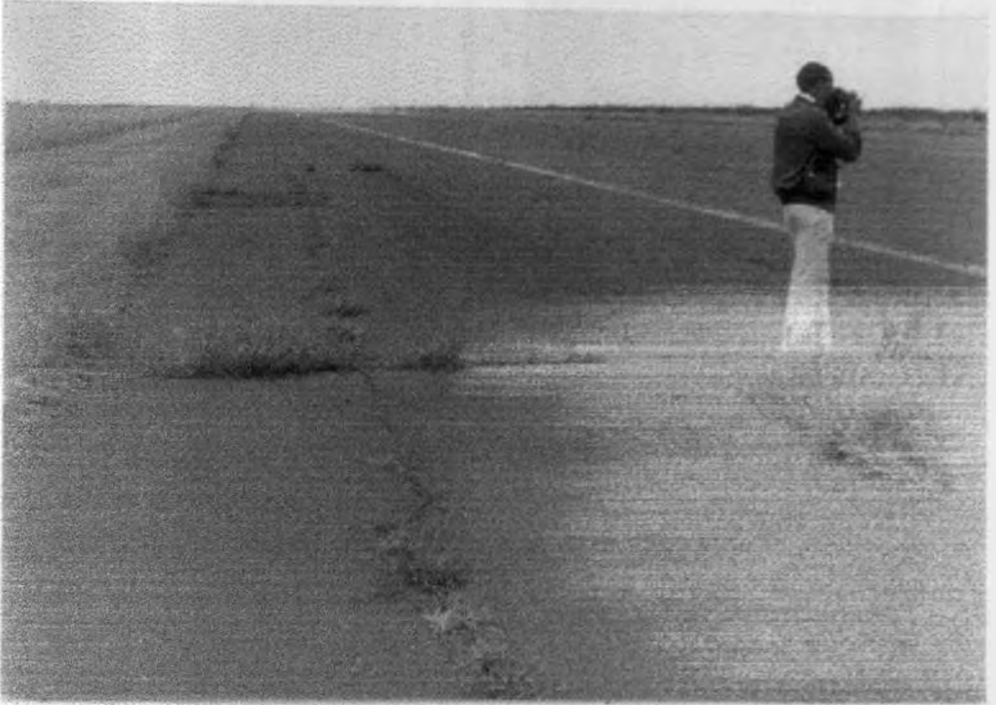
Plate A4.5 Weed growth on the pavements
