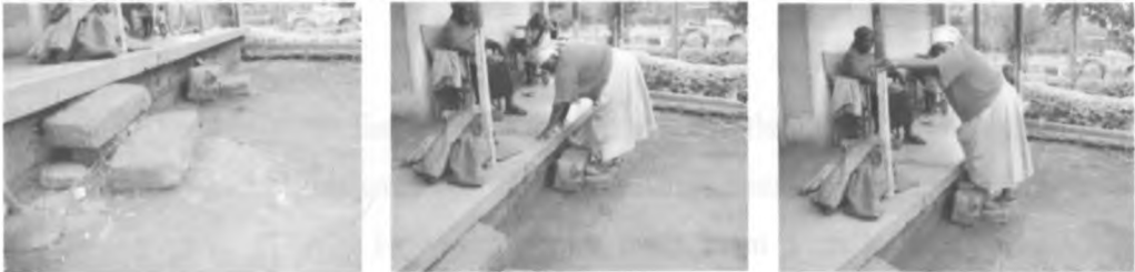
Figure 25: Wobbly Stairs Figure 26: A resident struggling to climb the stairs
