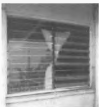
Figure 21: Missing panes in louver windows
