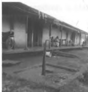
Figure 31: Dilapidated laundry at female hostel
