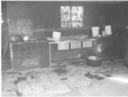
Figure 33: The flooring with poor drainage
