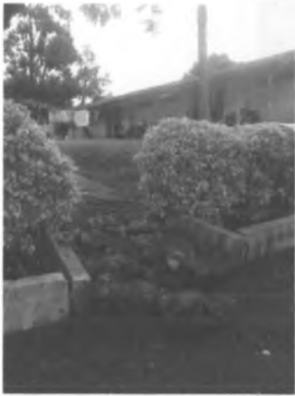
Figure 42: Hazardous entry to the female hostel
