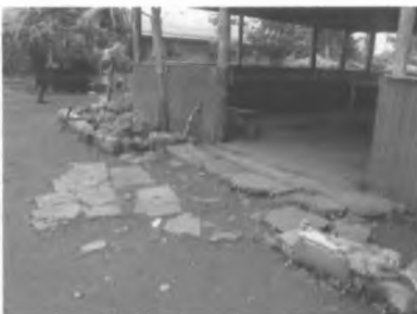
Figure 48: Uneven entrance acts as hindrance to wheelchair users
