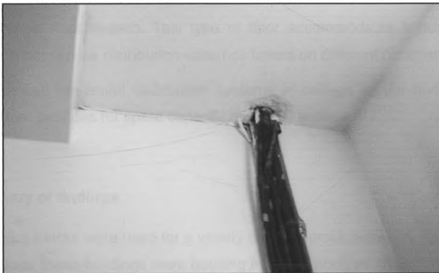
Plate 4.7: Power cables running through floor slab
