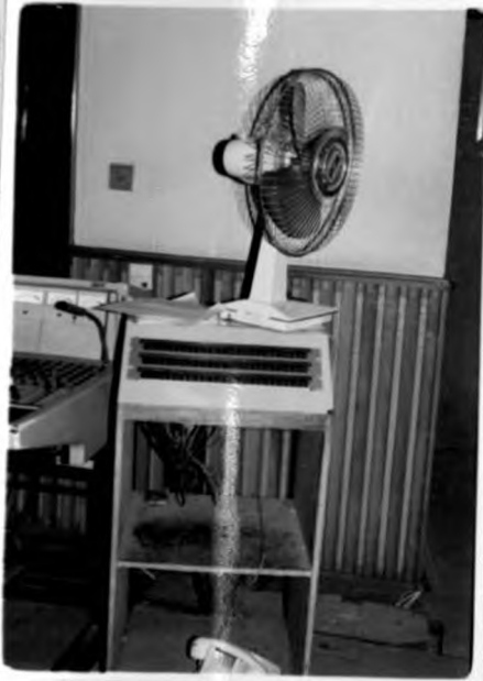
Plate 4.7 Studio's Control Room.
