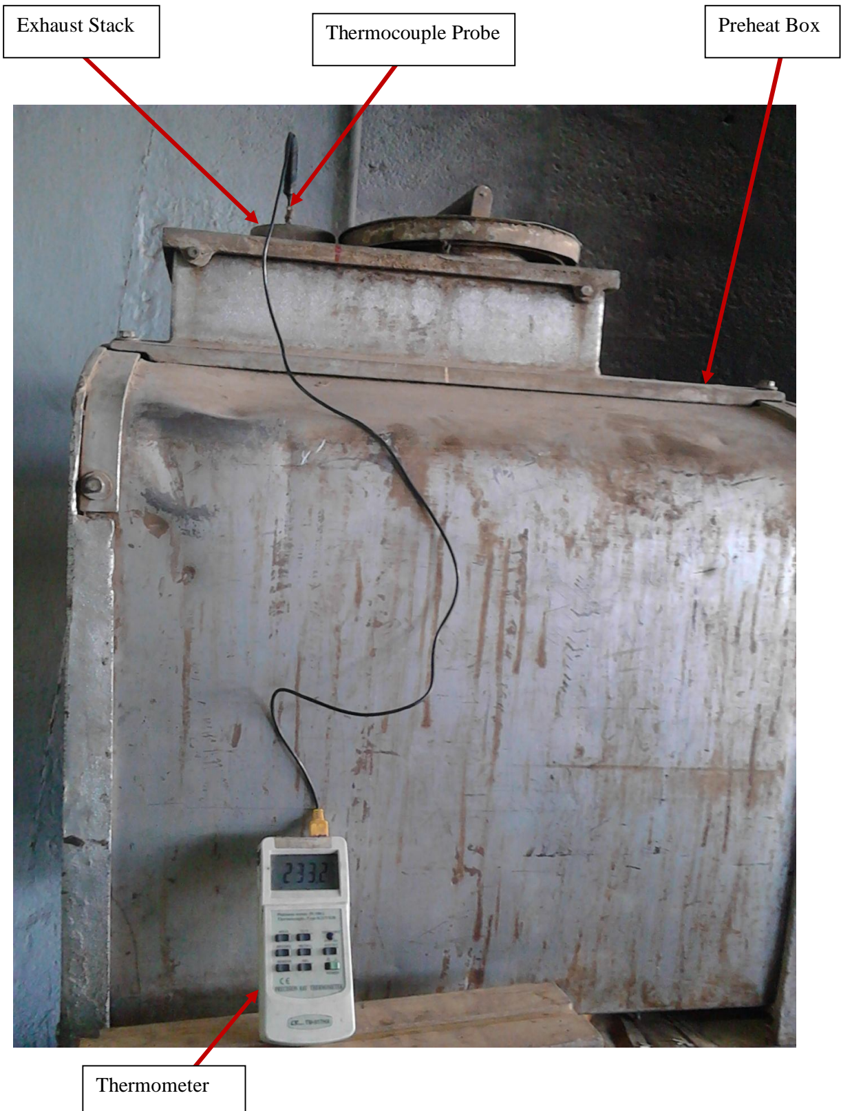
Figure 4. 6 Flue Gas Exhaust Temperature Measurement
