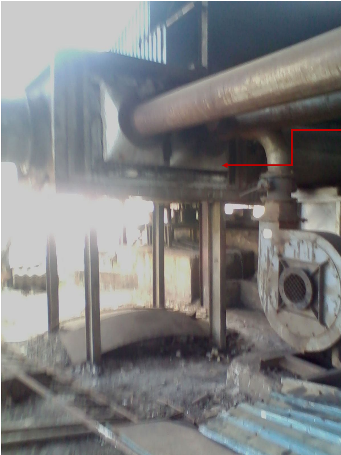
Figure 5.5 Recuperator not lagged
