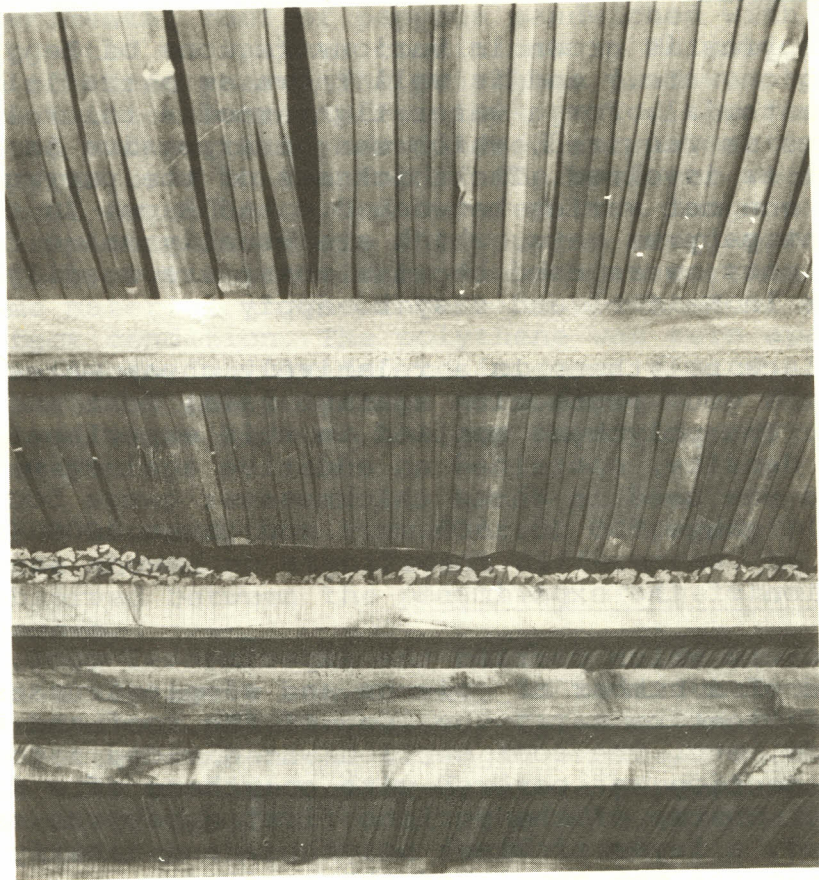
Photograph 2. Detailed picture of the method of sandwiching the polythene and papyrus mats. View of innerside.
